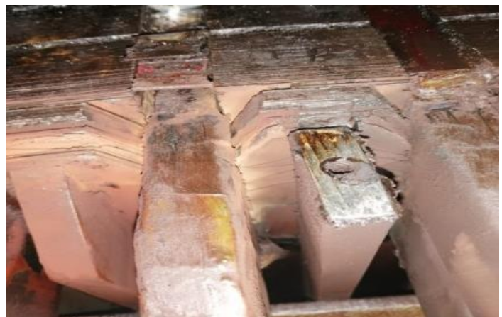
Figure 2. Burnt out Step Laminations
