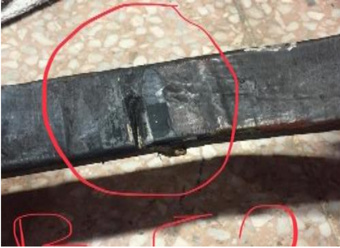
Figure 6. Damage on Bar due to Lamination Piece
